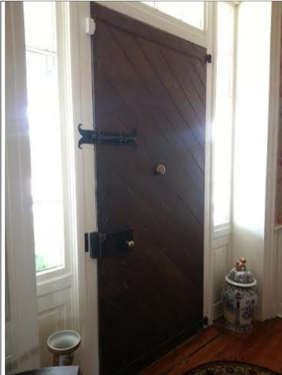
Fig. 17. Diagonally-braced door at main entry (front door). Built for strength and security, the door contains its original box lock.
